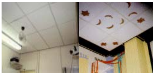
Detail of the ceiling, before (left) and after (right) the intervention of the volunteers. (Photo by Dr. Kevin Hope, University of Manchester, UK.)
